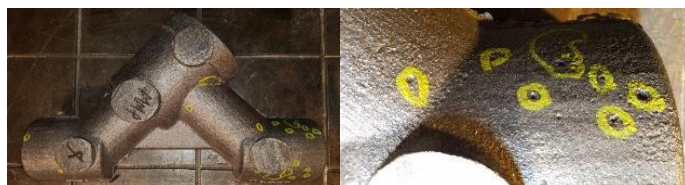
Inclusions Marked for Repair
